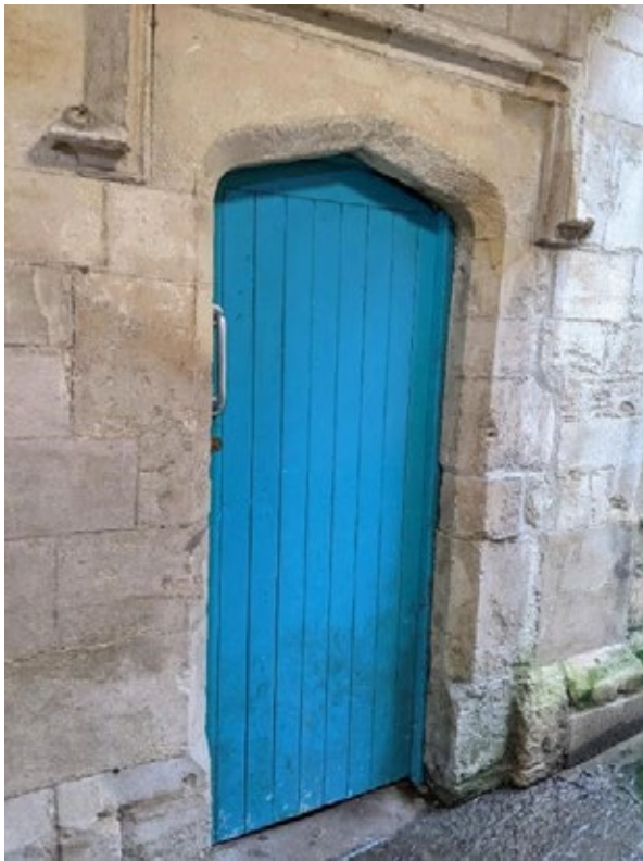
Figure 24: Door to old outside WC, in walkway under first floor kitchen
