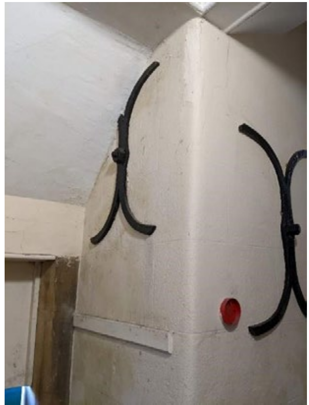
Figure 158: Staining on upper part of wall for internal emergency stairs
