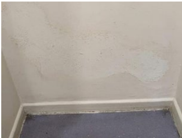
Figure 85: Water ingress into GF interior walls
