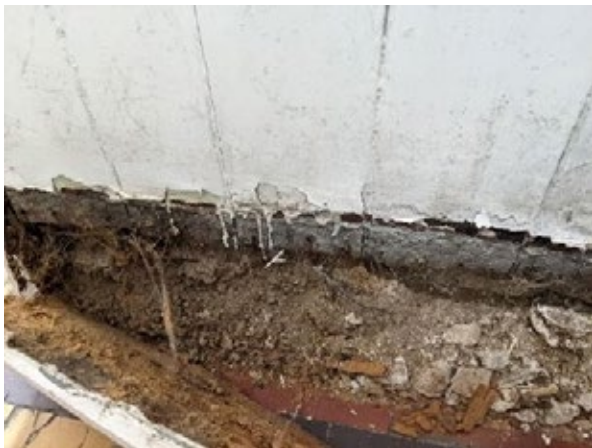
Figure 81: Behind loose skirting
