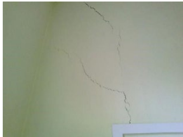
Figure 90: Photograph showing diagonal cracks in wall
