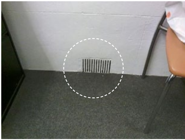
Figure 72: Photograph showing vent at bottom of north external wall in GF Office 3
