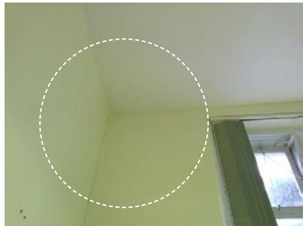
Figure 102: Photograph showing area at junction between roof, north wall and Office 2 partition wall
