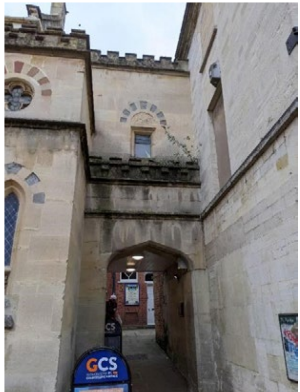
Figure 23: Archway and walkway under first floor kitchen, with vegetation growth in stone corncicing
