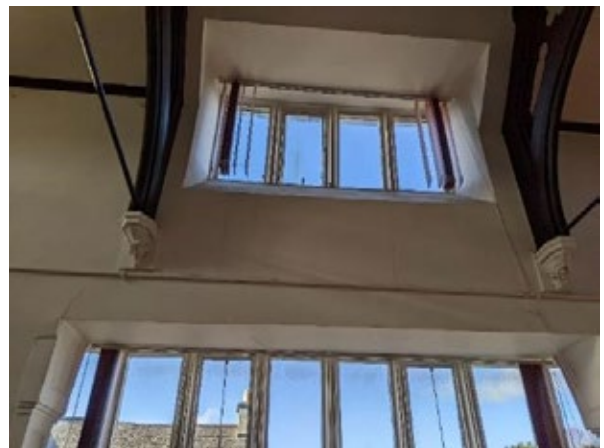
Figure 140: Water run marks from bottom of small window above main window of front (west) facing wall
