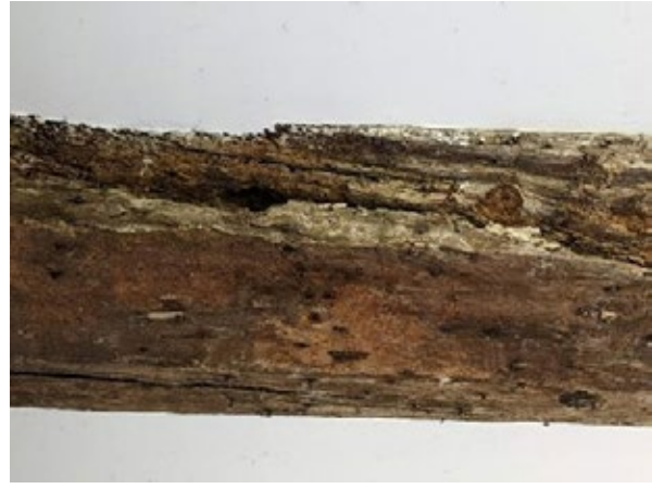
Figure 52: Evidence of timber decay
