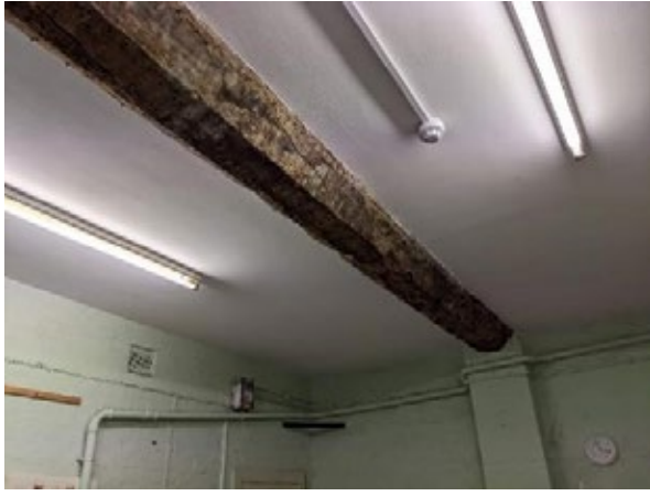
Figure 51: Timber beam in Store 4
