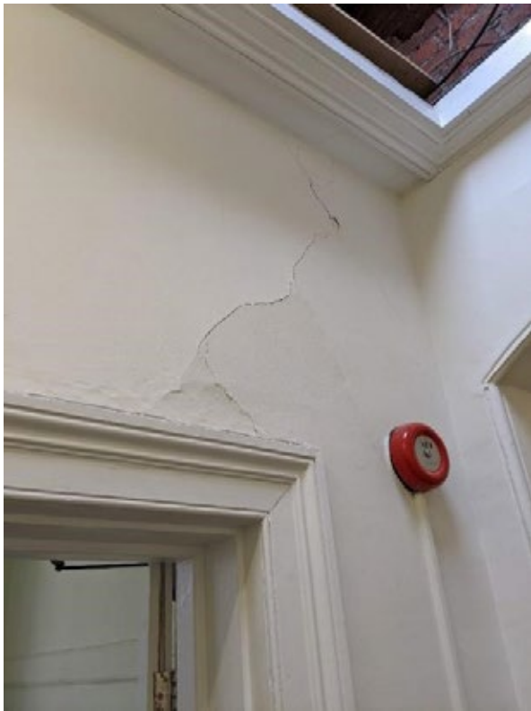
Figure 127: Diagonal crack above door to Office 5
