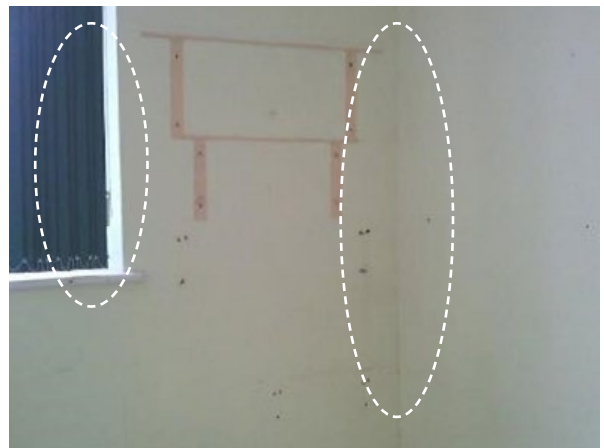
Figure 116: Photograph showing window reveal and external wall to partition wall junction next to Office 5
