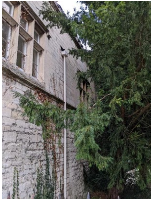
Figure 35: North wall, with extensive vegetation growth
