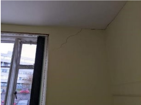
Figure 120: Diagonal crack in wall of FF Office 5
