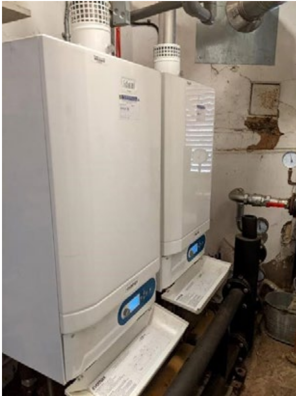
Figure 161: Mains gas boilers in plant room
