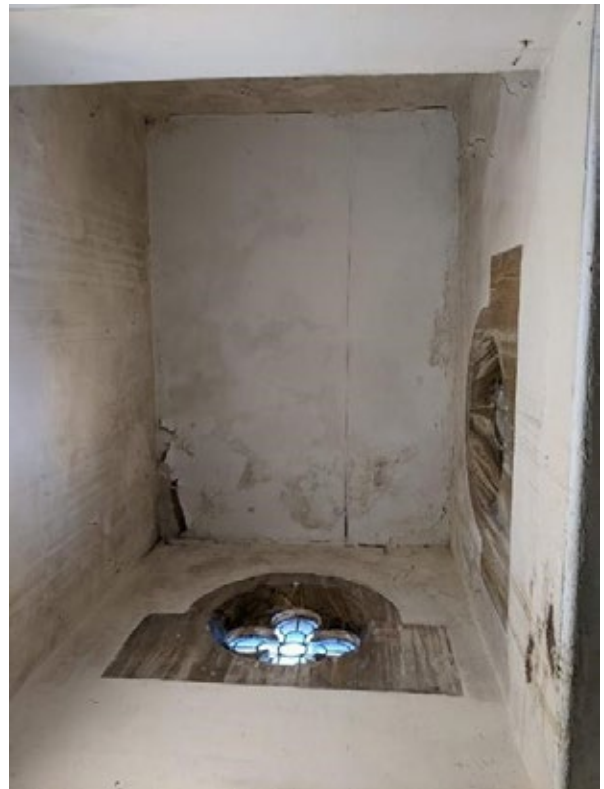
Figure 160: Significant staining to ceiling and upper walls above internal emergency stairs
