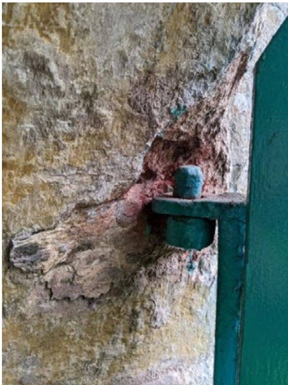
Figure 42: Store 2 entrance door hinge
