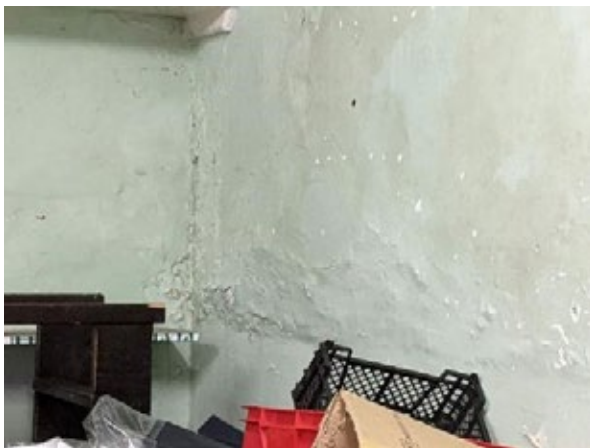
Figure 49: Blistering of plaster behind the paint
