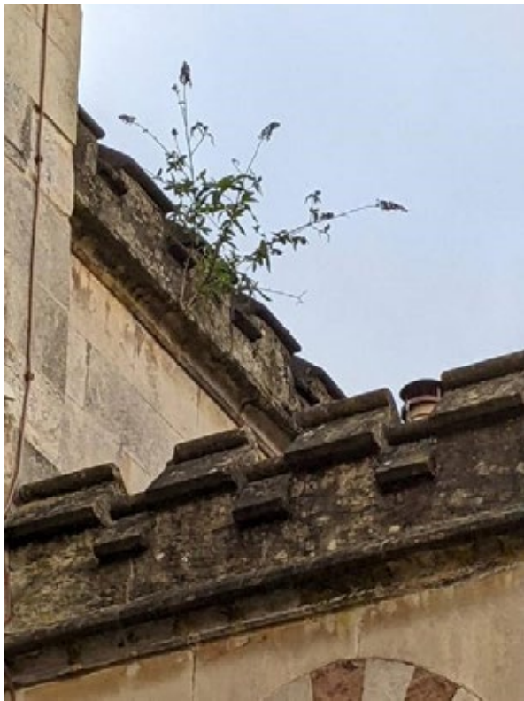
Figure 20: Vegetation growth in stonework of parapet, visible from front of the building
