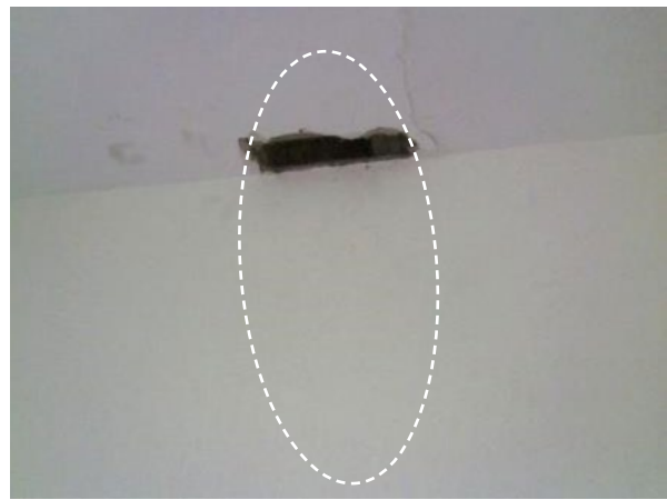
Figure 118: Photograph showing hole in ceiling in FF Office 4
