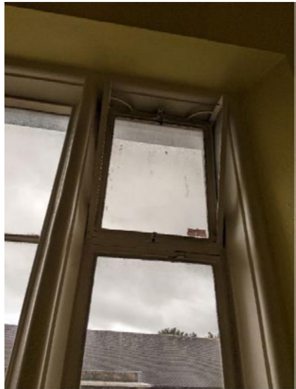
Figure 88: Top right of window, showing hinged openable section
