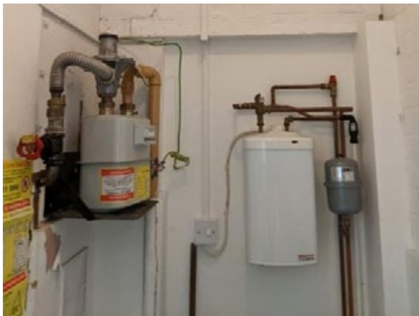
Figure 167: Mains gas meter and electric instantaneous hot water unit
