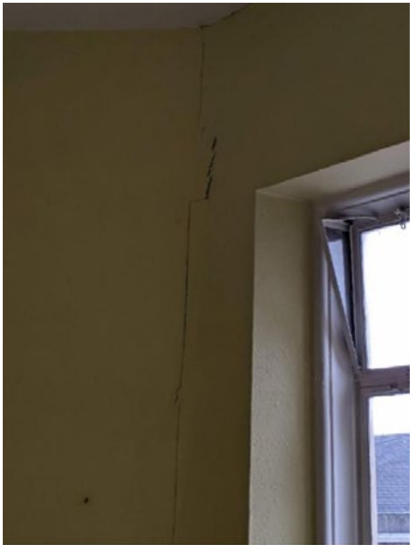
Figure 87: Vertical crack at junction between external wall and chimney breast
