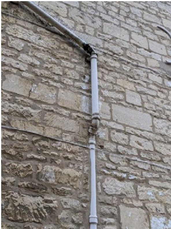
Figure 32: Rainwater pipe sunk into rear wall
