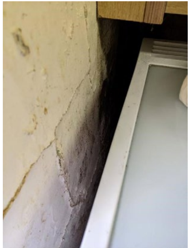
Figure 154: Wall behind fridge in kitchen
