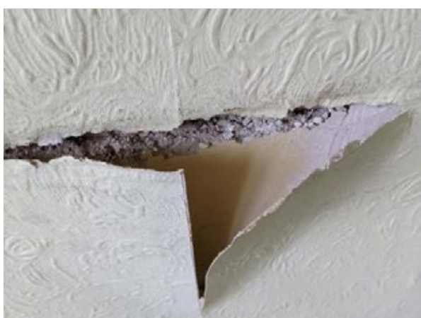
Figure 97: Damaged wall covering and plaster underneath
