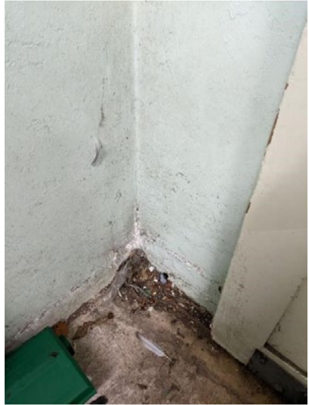
Figure 48: Salt crystals on surface of wall in corner
