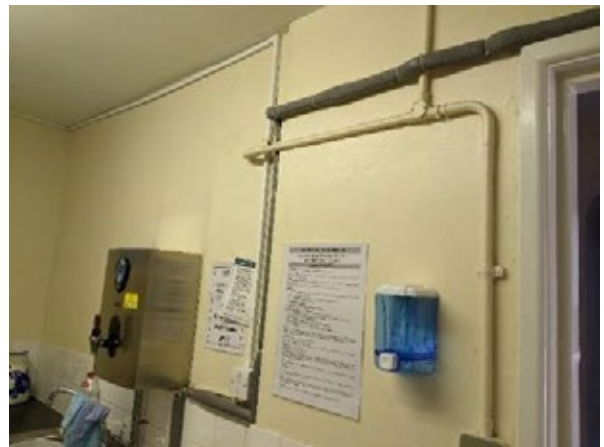
Figure 168: Electric instantaneous hot water unit and insulated hot water pipes
