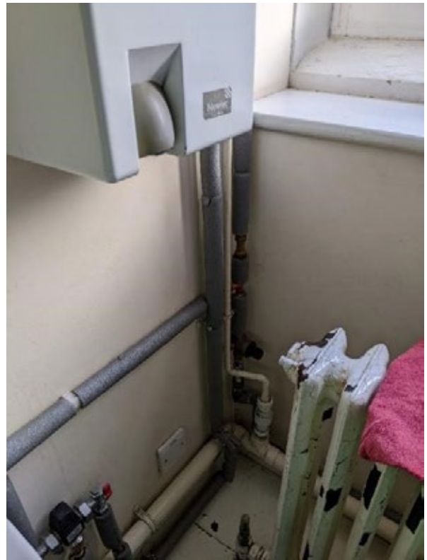
Figure 166: Insulated hot water pipes
