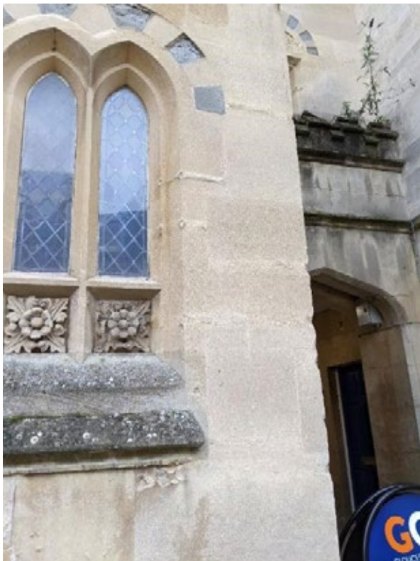
Figure 22: Blistering and delaminating stonework at the front of the building (near archway)
