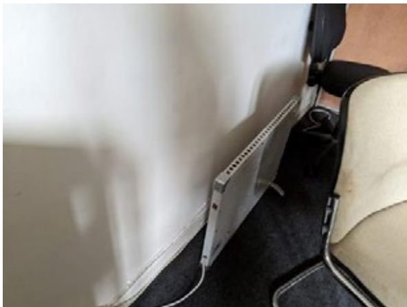
Figure 67: Electric heating panel in Office 2
