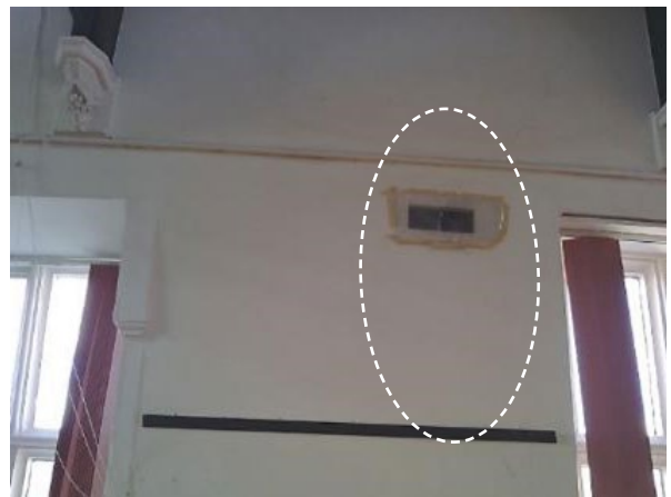
Figure 148: Photograph showing hole in the main façade wall (west facing)
