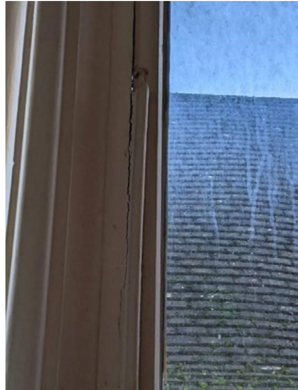
Figure 132: Crack in FF WC window frame
