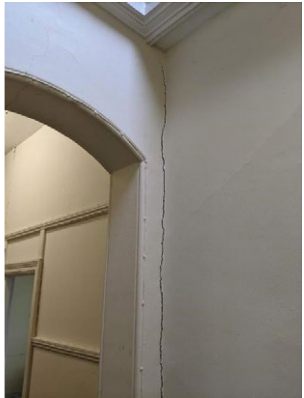
Figure 128: Vertical crack between cross wall and partition wall
