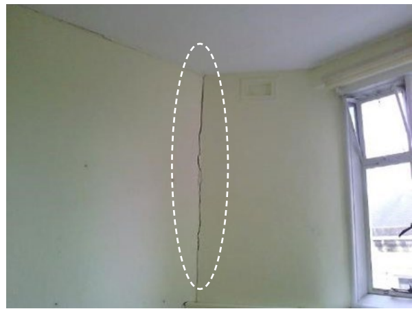
Figure 100: Photograph showing junction between chimney breast and partition wall for FF Office 1
