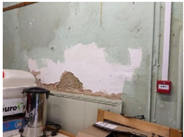
Figure 50: Delamination of the gypsum plaster
