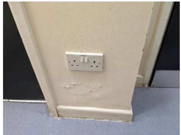
Figure 86: Water ingress into GF interior walls
