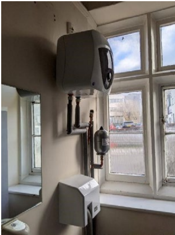
Figure 165: Electric instantaneous hot water unit
