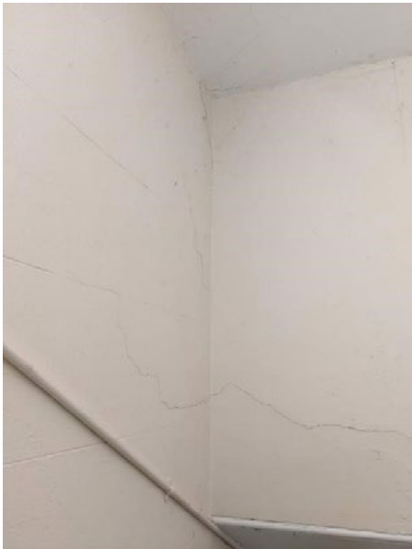
Figure 159: Cracks in paint and plaster on walls of internal emergency stairs
