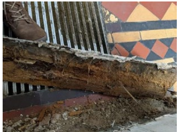
Figure 82: Back of loose skirting
