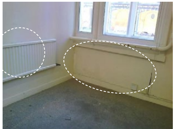
Figure 56: Photograph showing wall under window in GF Office 1
