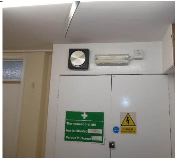
Photo 8 Mains electrical Cupboard
