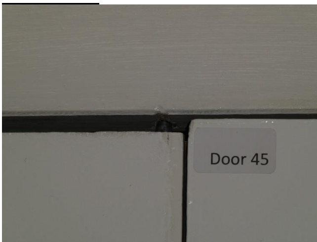
Photo 9 mains electrical cupboard gaps
