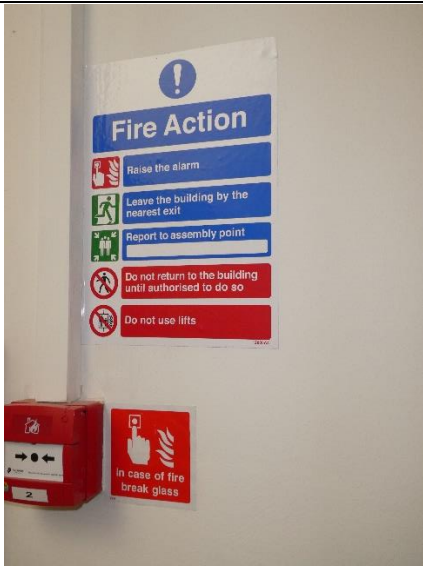
Photo 11 Incomplete information on FAN
