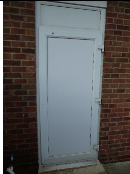
Photo 12 Missing Fire Door Keep Clear sign.
